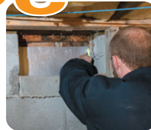
Blake Davis seals a major source of unwanted crawlspace moisture, the traditional foundation vent. Recent research shows crawlspaces should be sealed from outside air.
