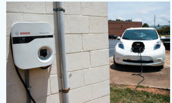
Walton EMC has installed a 240-volt aftermarket charging station for its Nissan Leaf. The professionally installed station charges the car in about eight hours. The 120-volt charging station included with the car takes about 20 hours to fully charge the vehicle.
